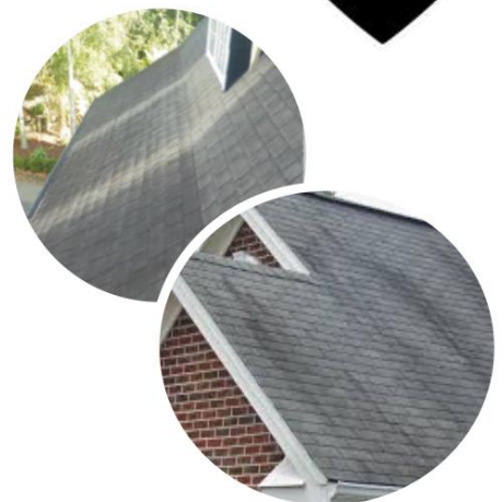
ALGAE STAINED ROOF
